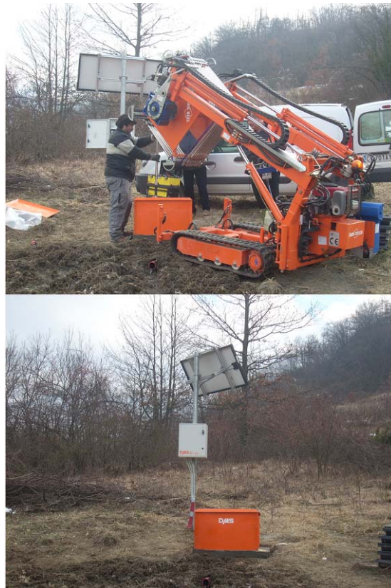
Figure 4.10-6. DMS 2011 during and after installation.
