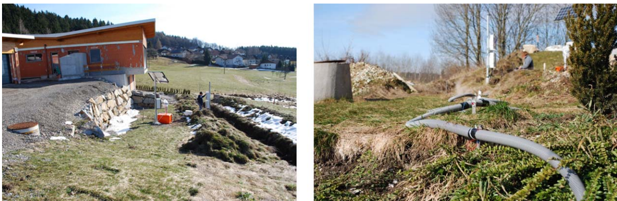
Figure 4.2-3. Situation at the Ampflwang monitoring site: DMS column located below the orange box and the trench with the GEOLMON 4D cables (left) and part of the cable situated on the ground surface (Photo: Ivo Baroň).
