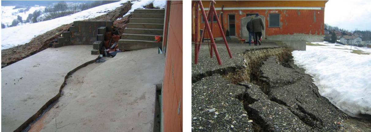
Figure 4.2-2. Damage of a newly constructed house caused by the shallow landslide in March 2010. The landslide has been monitored since then for displacement and geoelectric parameters (Foto: J. Gaisbauer)
