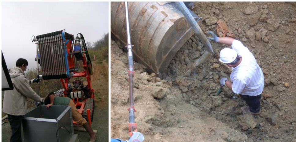
Figure 4.4-3. DMS column installation (October 28 th 2008) and removal (July 13 th 2009) - Bagnaschino site (Photo: C.S.G.).
