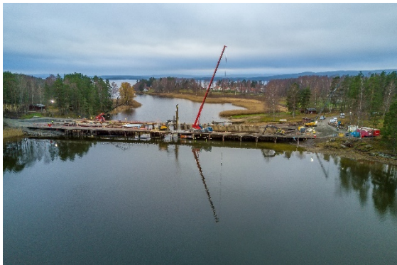
Figure 6. Drone photo of the construction of a new flood protection dam (photo: NRC Group).
